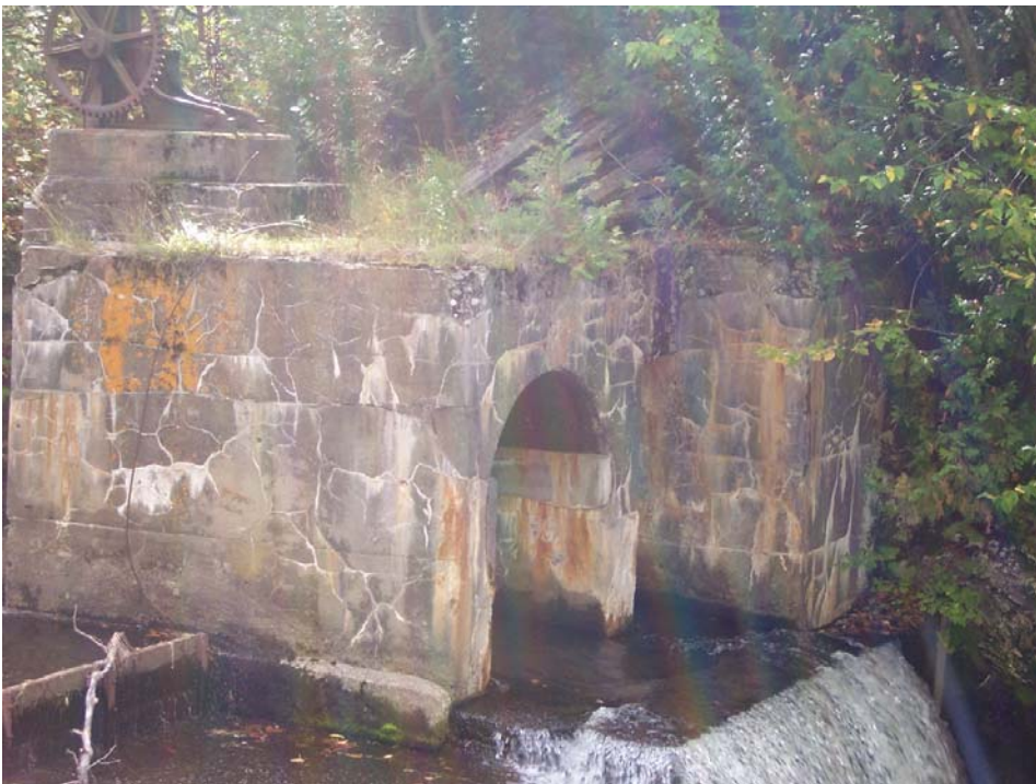
Photo No. 2 – View of the low-level slide gate at the left abutment of the dam. The 45 cfs minimum flow is currently being released through this gate.
