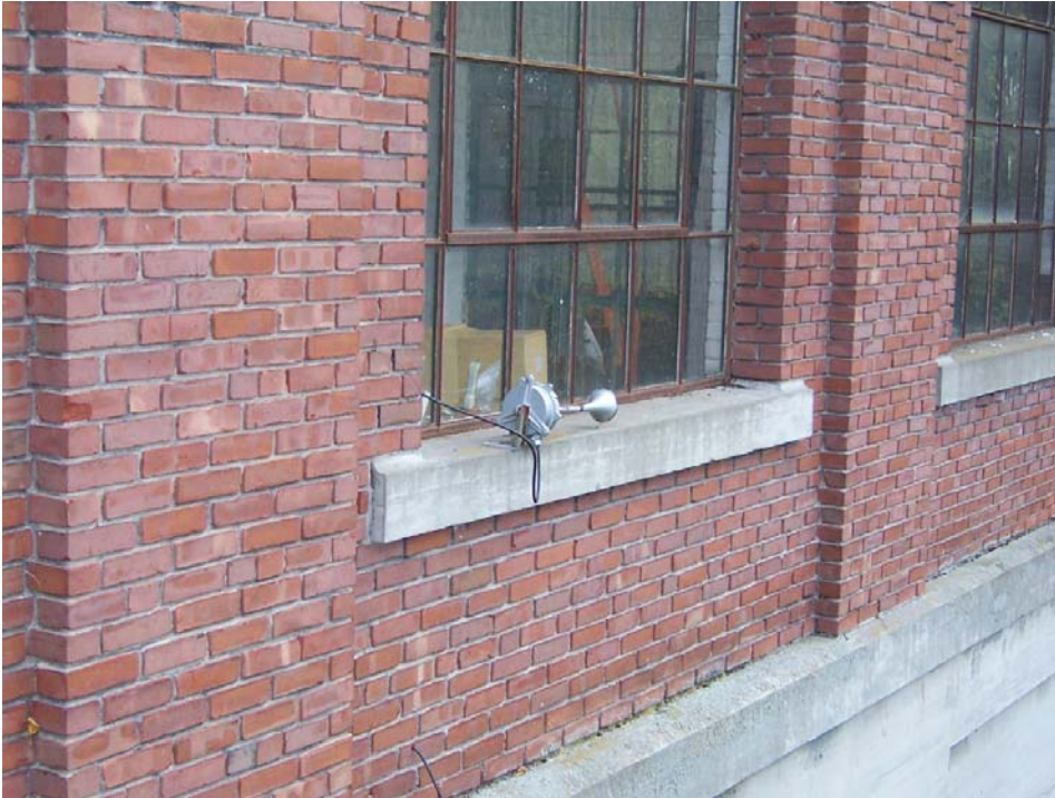
Photo No. 5 – View of the horn to warn fishermen and boaters mounted on the window sill on the tailrace wall of the powerhouse.
