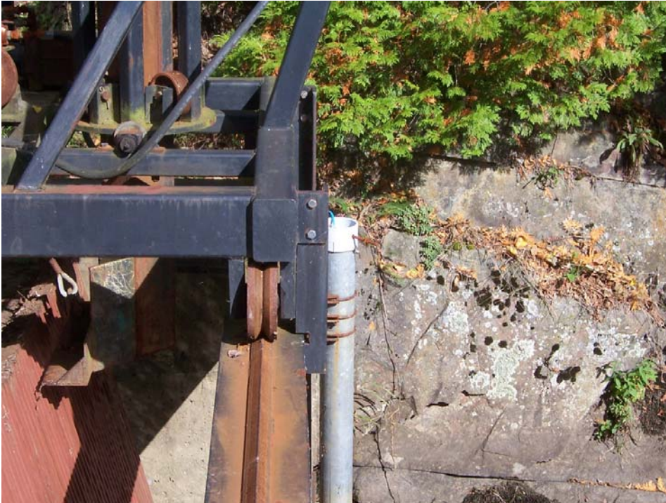
Photo No. 3 – View of the headpond level sensor in front of the trashracks and intake. Note mechanical trashrake in front of the trashracks.
